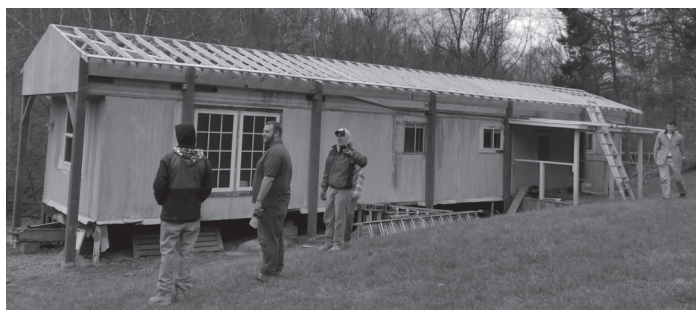
Shelli's new roof over during an April Group Week with St. John's & Xaverian Brothers
